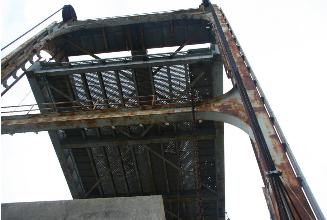
Condition Photo 10: West lift tower with bridge open; note holes in metal sidewalk plates.
