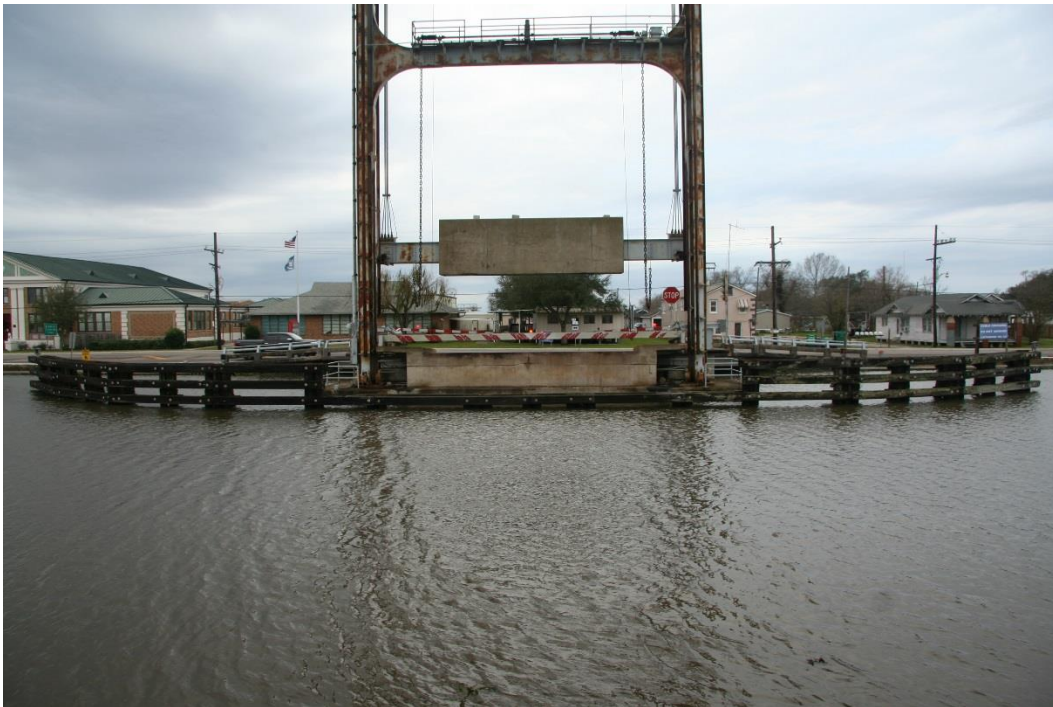
Condition Photo 7: West lift tower pier and timber fender system, looking west.
