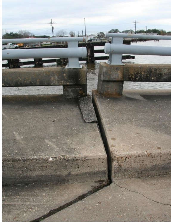
Condition Photo 14: Sidewalk and deck joint in southwest quadrant of west approach span.
