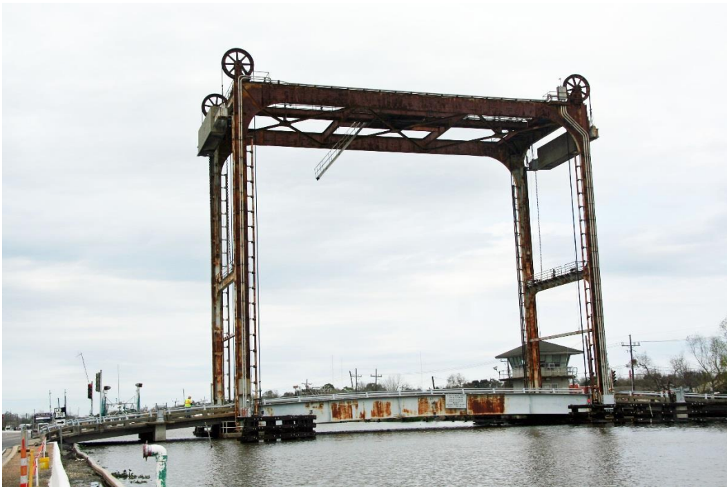
Condition Photo 9: Elevation view of south side of bridge, showing bridge and navigation channel.
