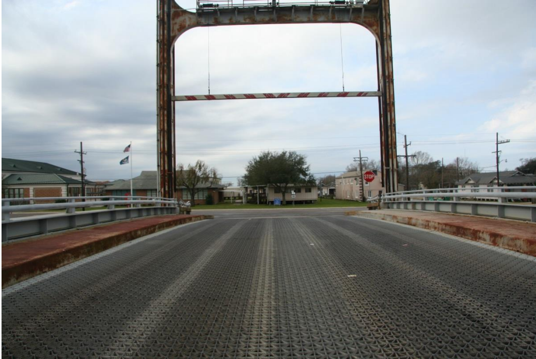
Condition Photo 1: Looking west from center of bridge at LA 1 intersection on west side of bridge.
