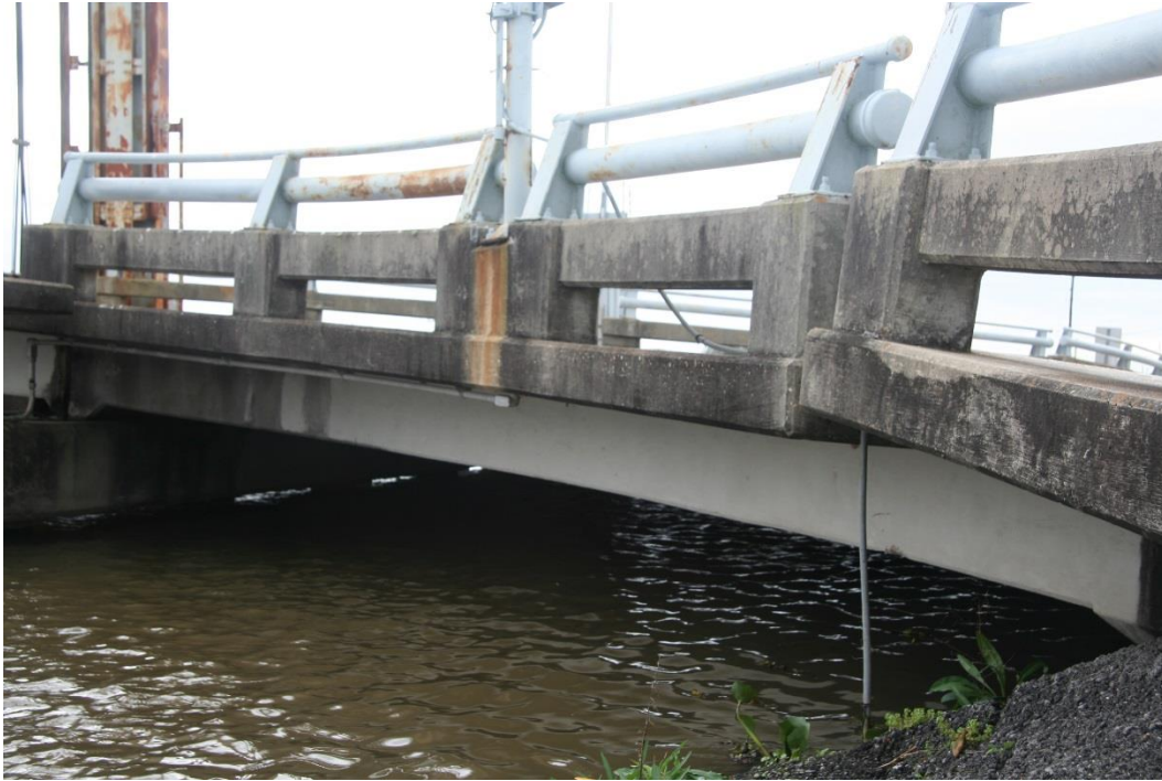
Condition Photo 18: North side of west approach spans; note misalignment in railing.
