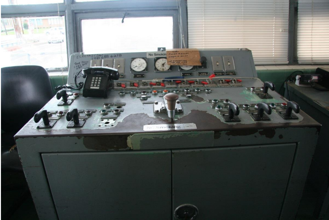
Condition Photo 16: Control panel and inside of bridge operator's house (second floor).
