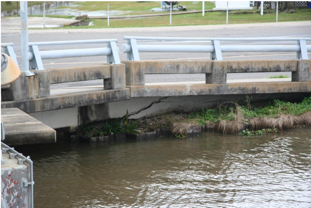
Condition Photo 19: South side of east approach spans; note large diagonal crack.
