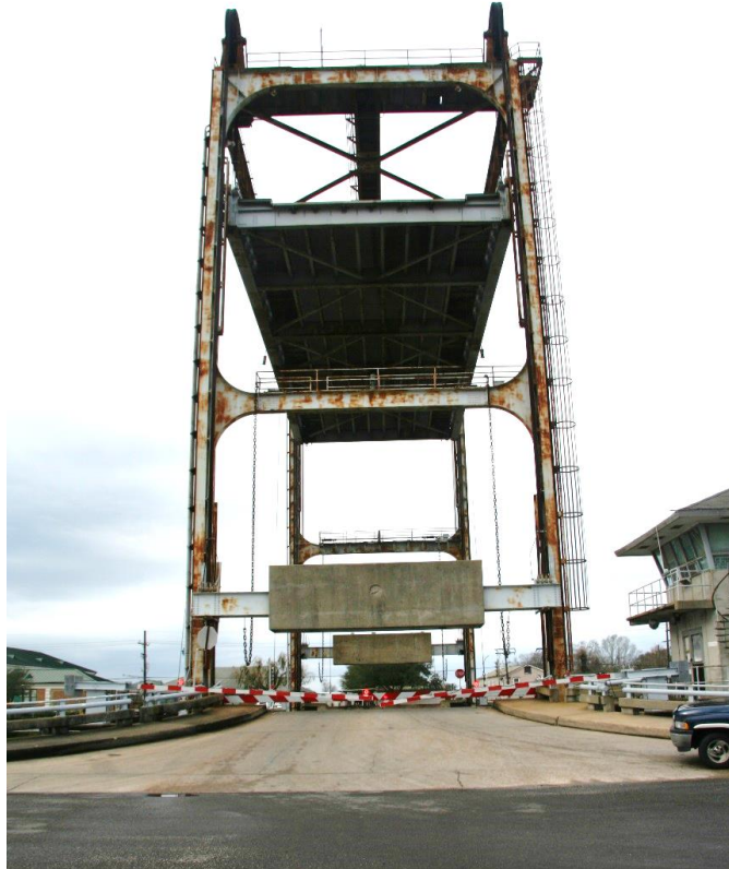
Character-defining feature Photo 2: Vertical lift span with central drive machinery, with the platform raised, as seen from LA 308.
