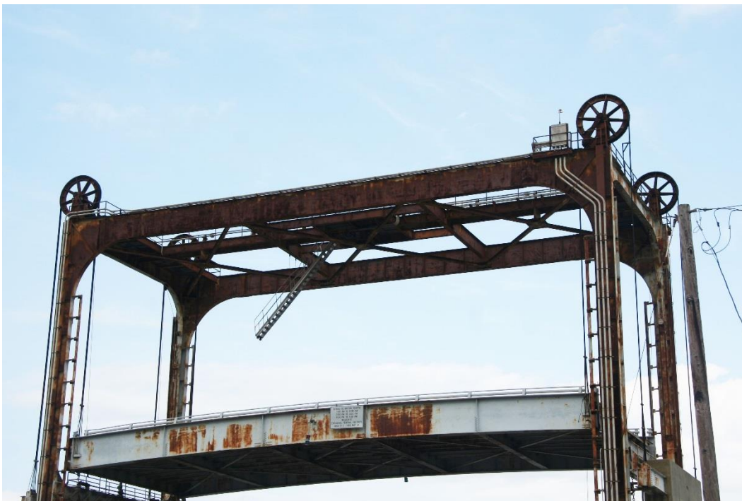
Condition Photo 3: Lift span in open position; note failed paint system on lift span and towers.
