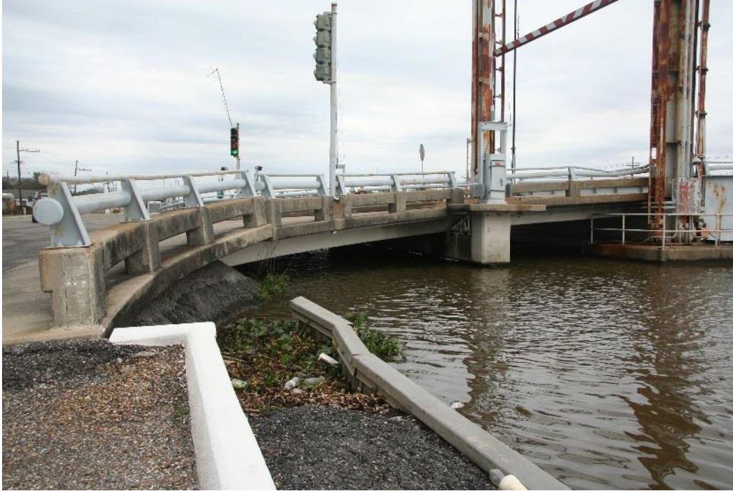
Historic Fabric Photo 3: Approach spans with concrete piers, abutments, curbs, sidewalk, and railing, on southeast side of the bridge.
