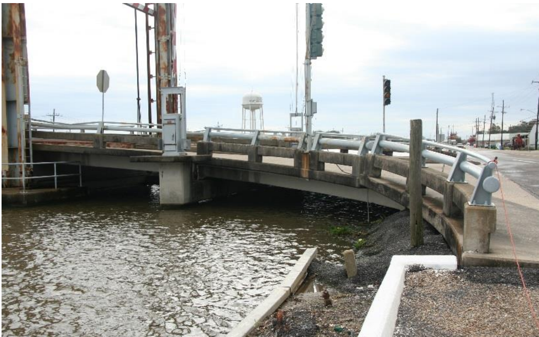
Historic Fabric Photo 2: Approach spans on the northwest side of the bridge including concrete piers, abutments, sidewalks, curbs, and railing. Metal railings have been added to the top of the concrete railings, a minor alteration that does not affect the bridge's significant features.
