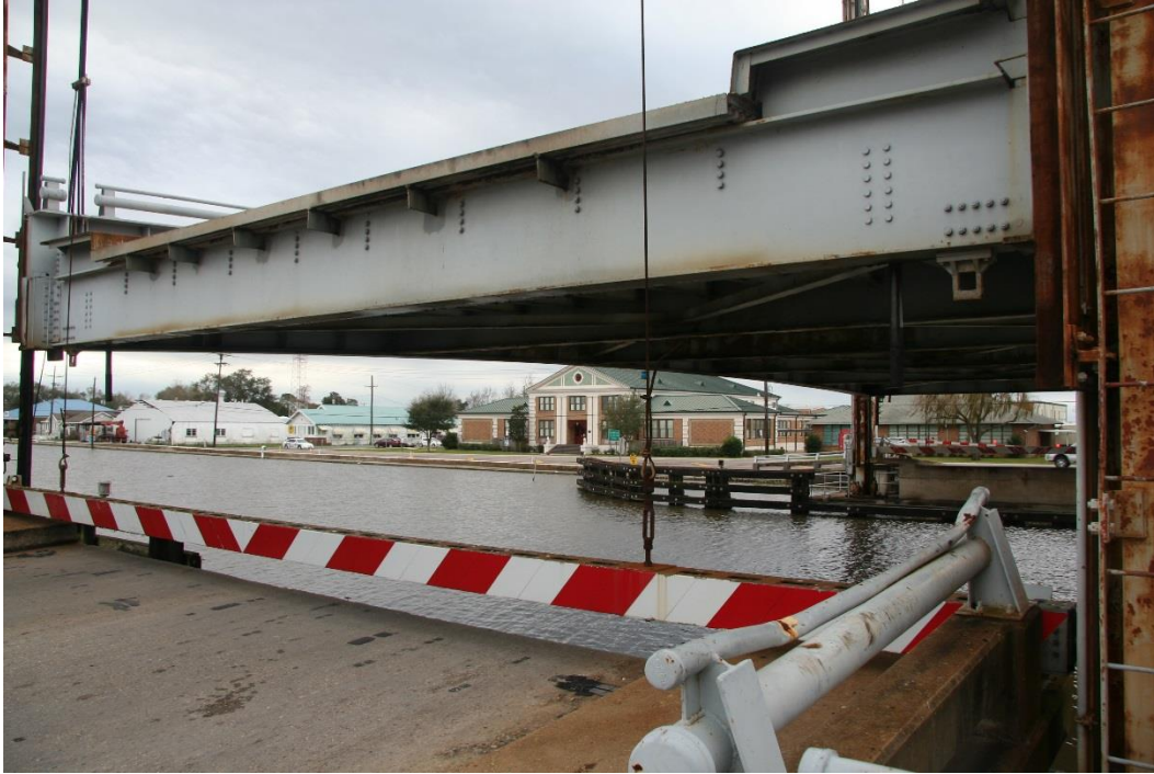
Condition Photo 8: West end of lift span; condition of damaged tubular bridge railing; traffic barrier gate is down.
